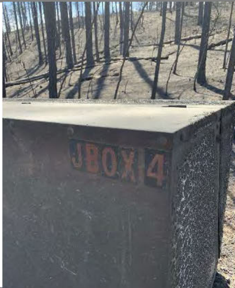
0253 Aspect SW, junction box labeled "JBOX 4" on FS road 10DD
